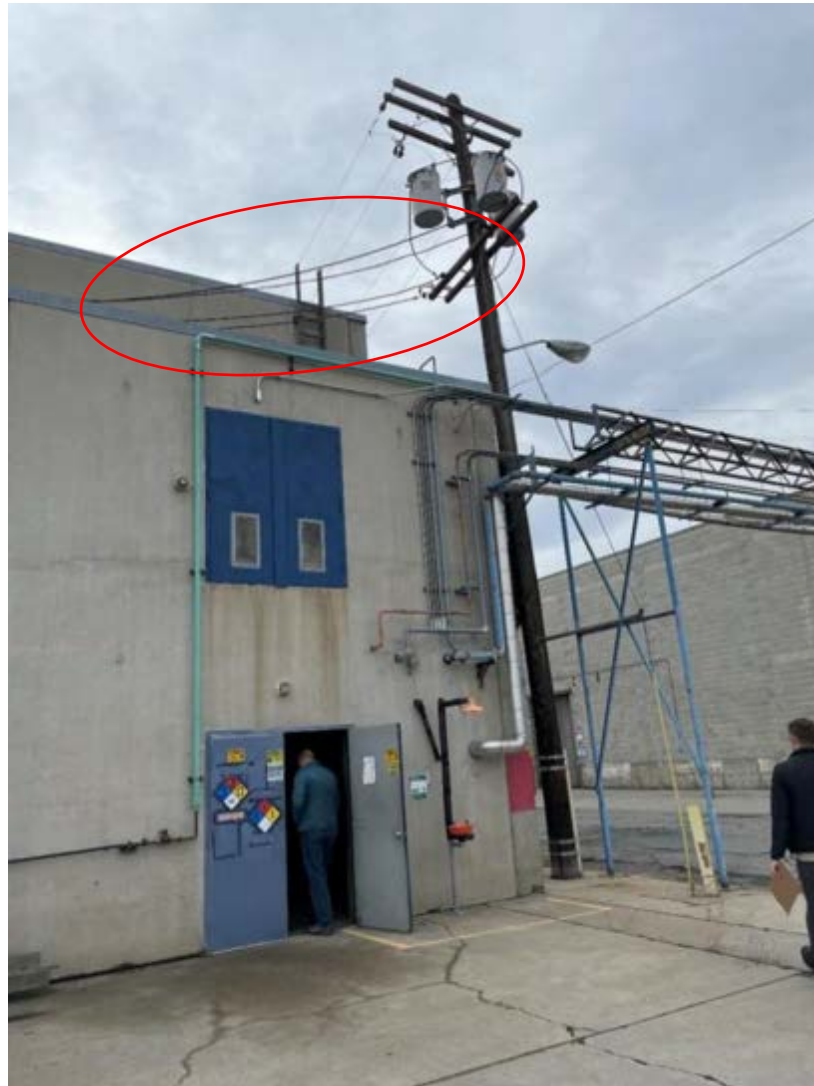
Figure 21: Building F Utility Service Drop
