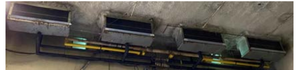
Figure 5: Ammonia Refrigerator Units
