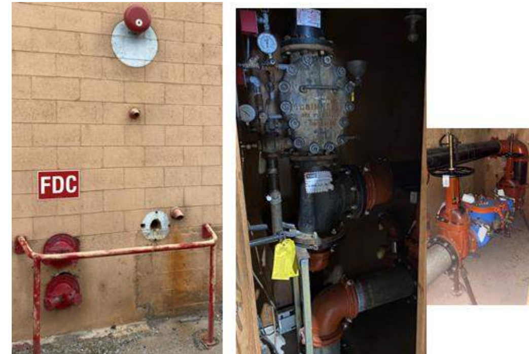
Figure 13: Building D Fire Department Connection, Backflow Preventer, and Riser
