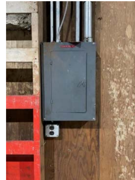
Figure 19: Existing Branch Panel in Building D
