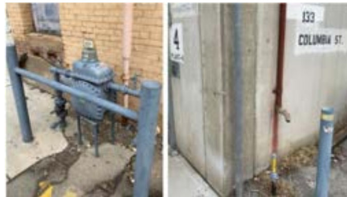
Figure 9: Building B Gas Meter and F Meter Location
