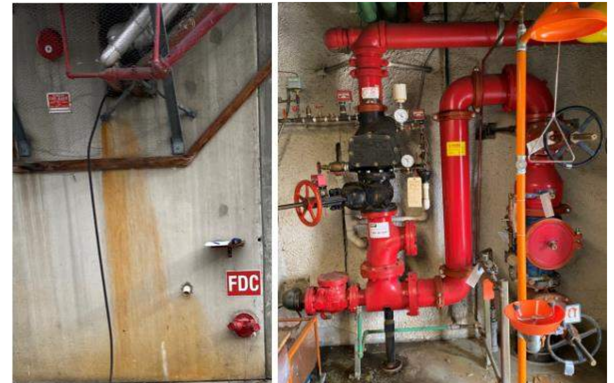
Figure 14: Building F Fire Department Connection, Backflow Preventer, and Riser
