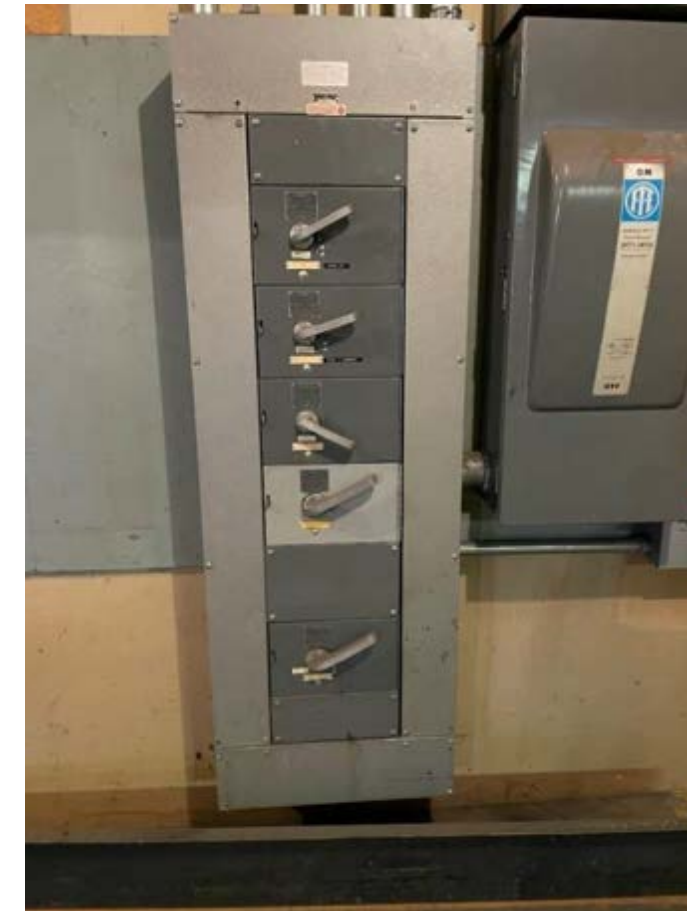
Figure 18: Building C Level 1 Distribution Panel
