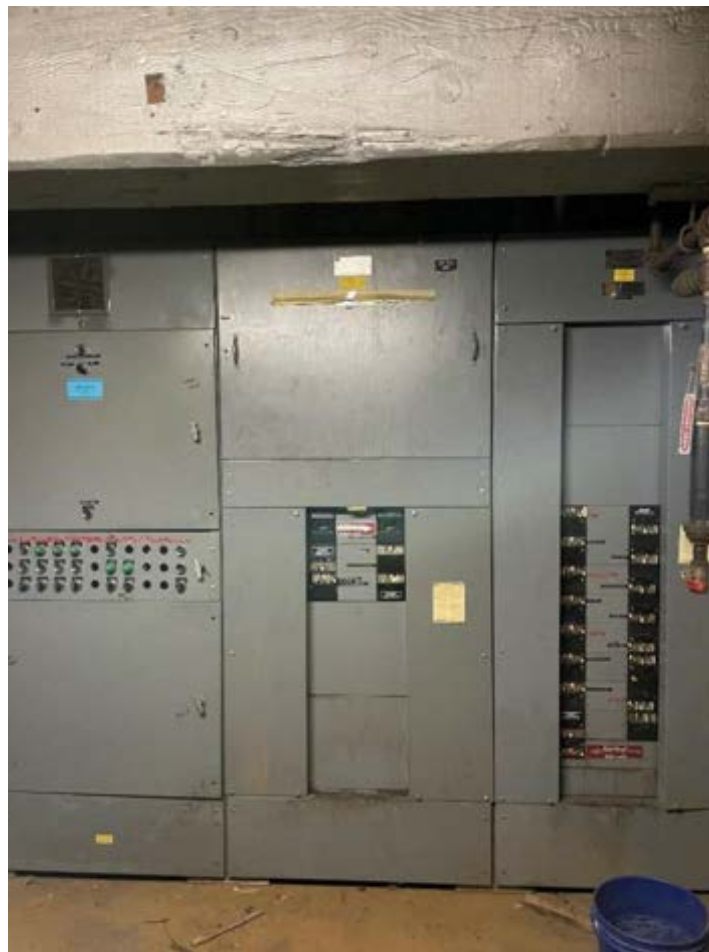
Figure 17: Building C Basement Main Distribution Panel
