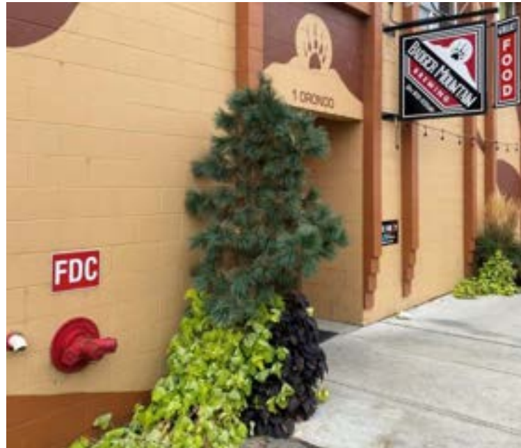
Figure 11: Building A Fire Department Connection, Backflow Preventer, and Riser
