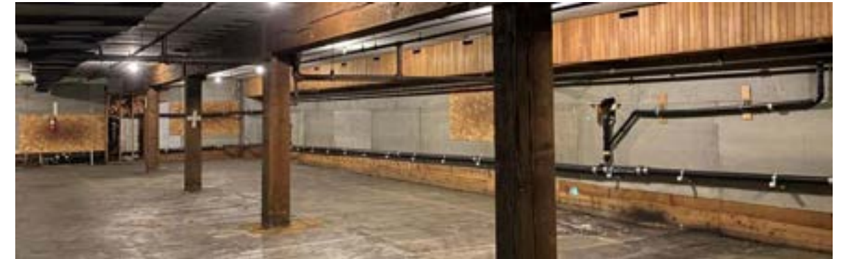
Figure 8: Building B Lower Level Sanitary Piping
