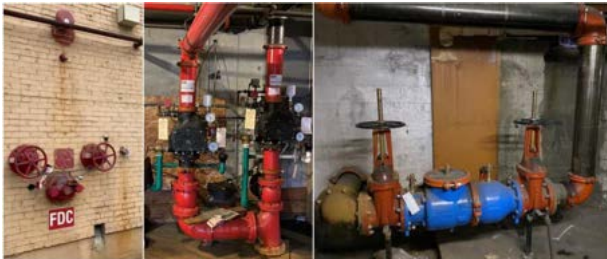
Figure 12: Building C Fire Department Connection, Backflow Preventer, and Riser
