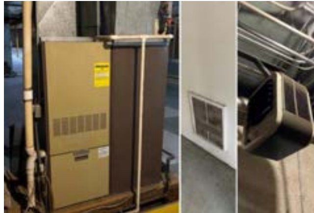
Figure 3: Building B Furnaces, Building D Wall Heater, Building F Unit Heater
