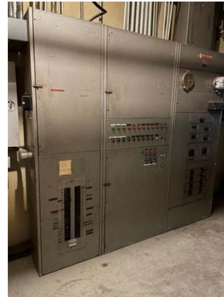
Figure 20: Building F Main Switchboard and Meter
