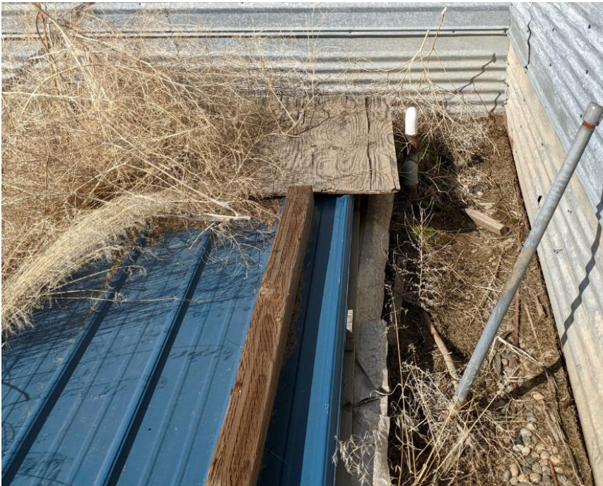
Photo 7 – Closeup view of SE building corner. Note 2" PVC vent pipe in upper righthand corner indicating the possible present of a underground storage tank. Could not determine if galvanized pipe is connected. Steeling siding appears to be stored on a concrete pad.
