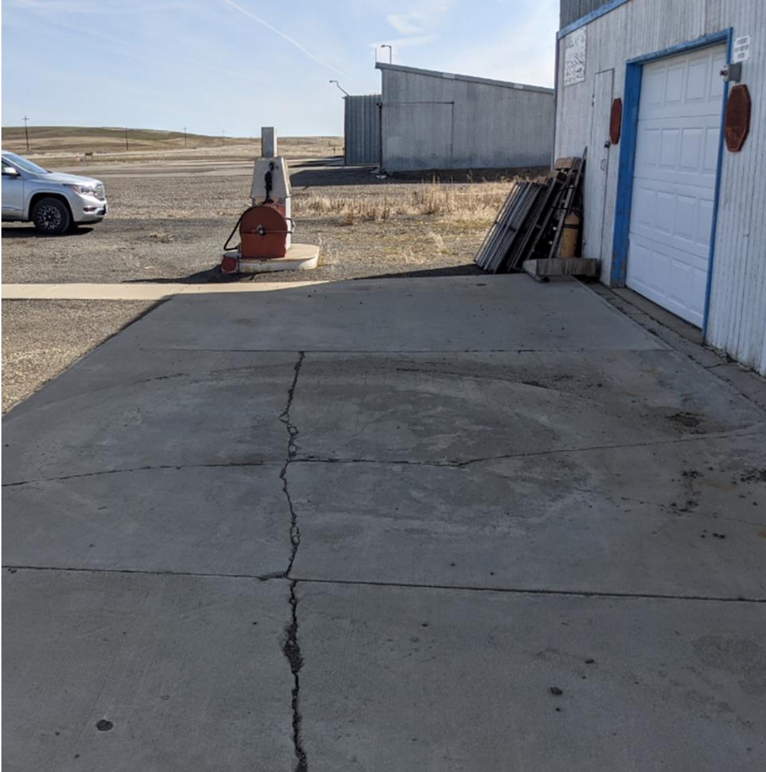
Photo 10 - View to the east showing fuel dispenser and concrete apron along the front (airside) of the building. Note circular staining of concrete apron with unknown chemical. The Concrete is in poor condition with significant cracking and surface deterioration and pocking indicating the use of deicers or other chemicals.
