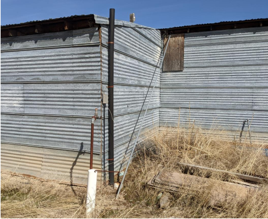
Photo 6 – Closeup of SE building corner. White PVC pipe with rebar valve handle and galvanized pipe appears to be domestic water supply (for unknown use - chemical mixing?). Black ABS pipe on side of building appears to be a waste vent pipe indicating a possible septic tank and drainfield.
